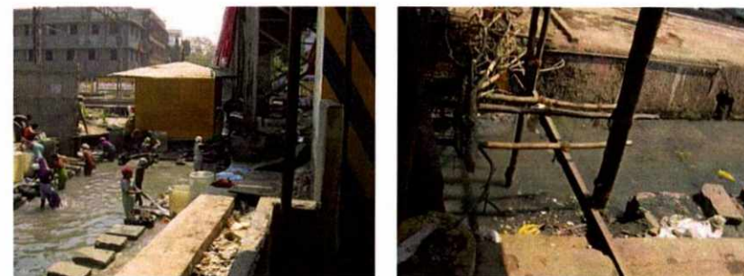
Figure 2.8: MMR – Existing Drain Conditions Source: Surbana
