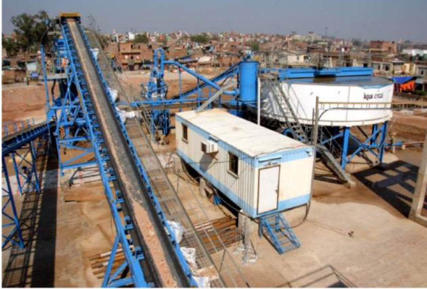
Crushing units at Burari C&D waste recycling plant
